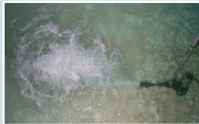
▶ Submersible Ejector Pump job site
